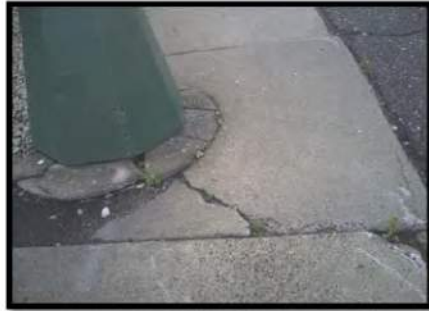
Traffic Signal Pole
