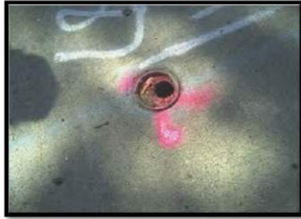
Water Gate Valve
