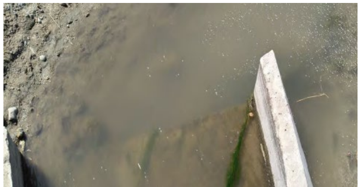
A culvert that may be a fish barrier (Stressor Identification Report)
